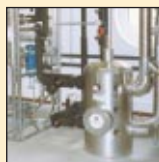
Wasser-Ammoniak-AKM in Köthen
